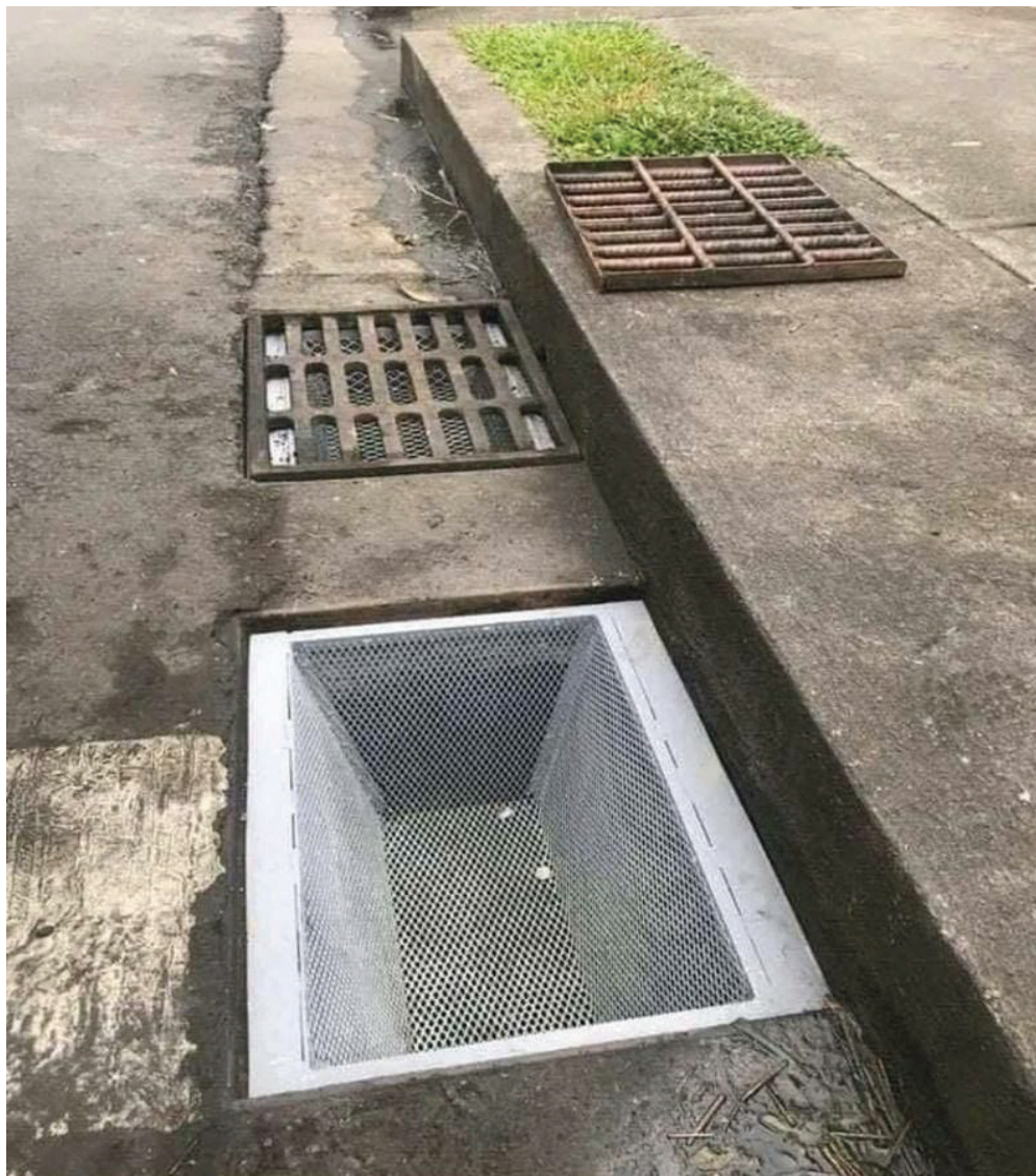
Fig. 6.10 Filtration over Smart Tank
