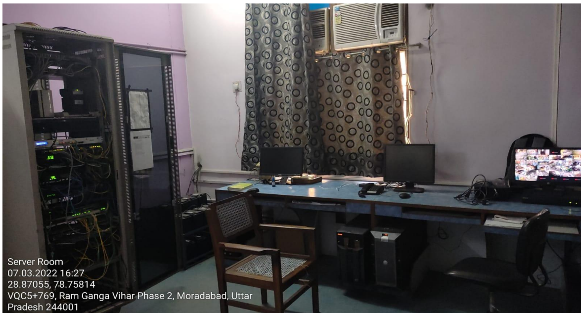
Image 10: Server Room (Firewall and other Related Network Devices)
