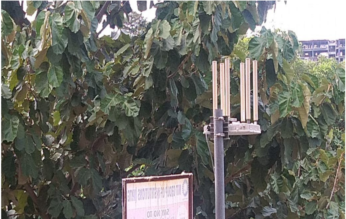
Image: WIFI Access Point
