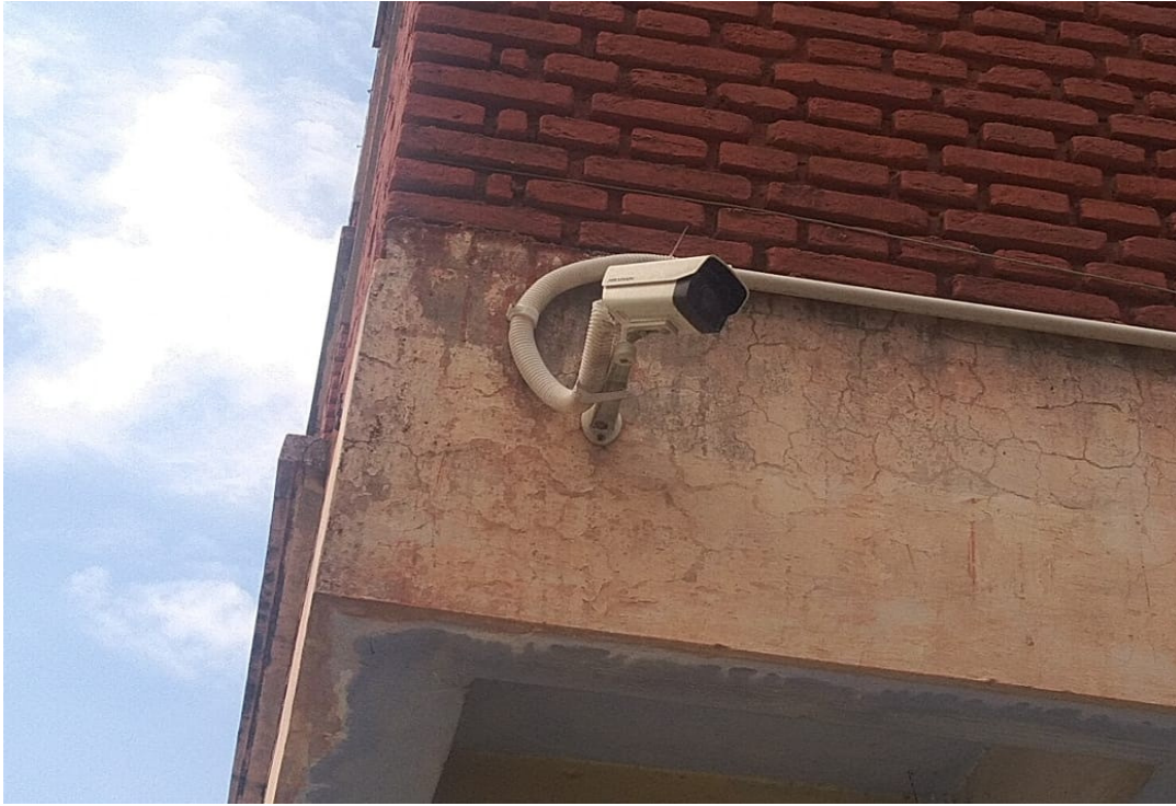
Image: Cameras Installed at Various Places
