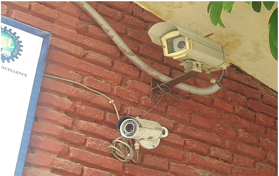
Image: Cameras Installed at Various Places
