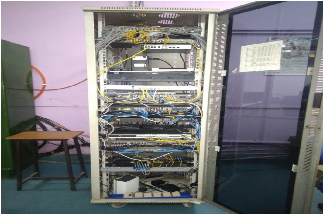
Image: Server Room (Firewall and other Related Network Devices)
